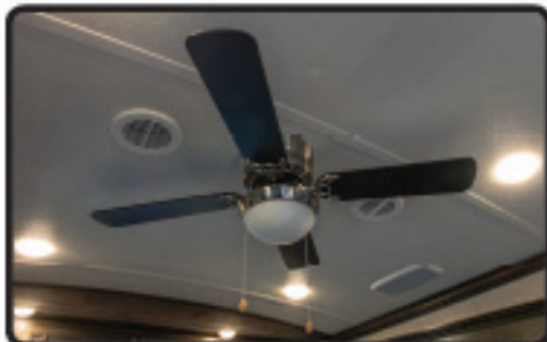
RESIDENTIAL CEILING FAN PROVIDING NATURAL AIR MOVEMENT
